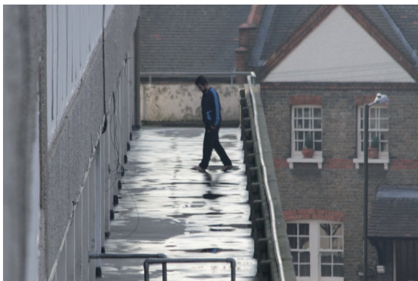
Fig.4.14 Unpopular deck access and failing elevators were major issues in high rise blocks. (Photo: Mattia Marinoli, 2013)
