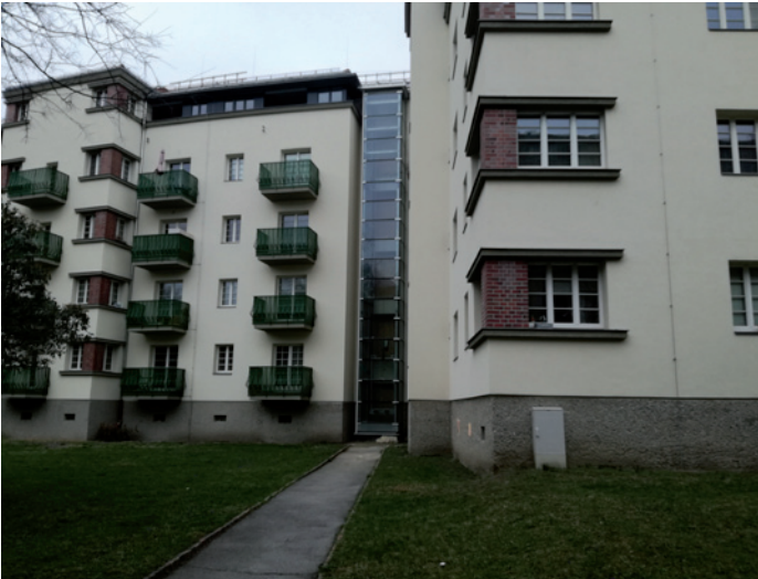
Fig.5.19 Renovation of the Goethehof: thermal improvements, addition of balconies, elevators and an additional storey (Photo: author)
