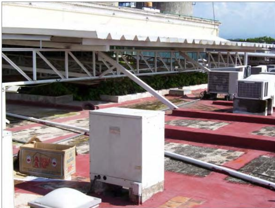
Figure 11.32. Roof of the patio with timber slats below translucent roofing sheets on an open structure to achieve good ventilation.
