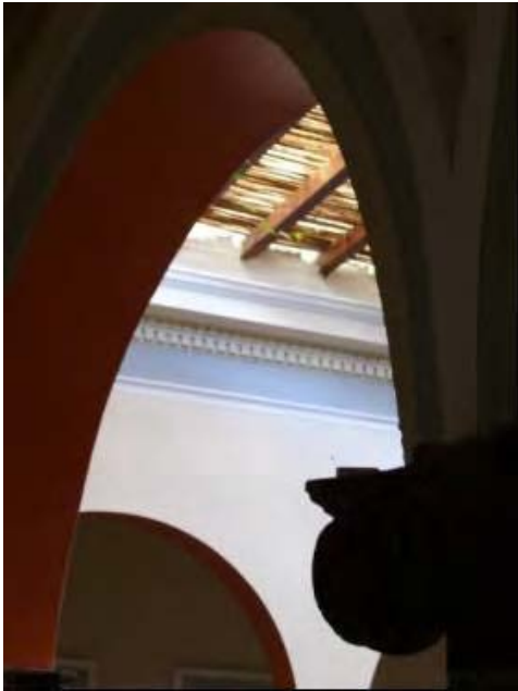
Figure 11.30. Roof of the patio. Location of the HOBO sensor placed on the capitel.
