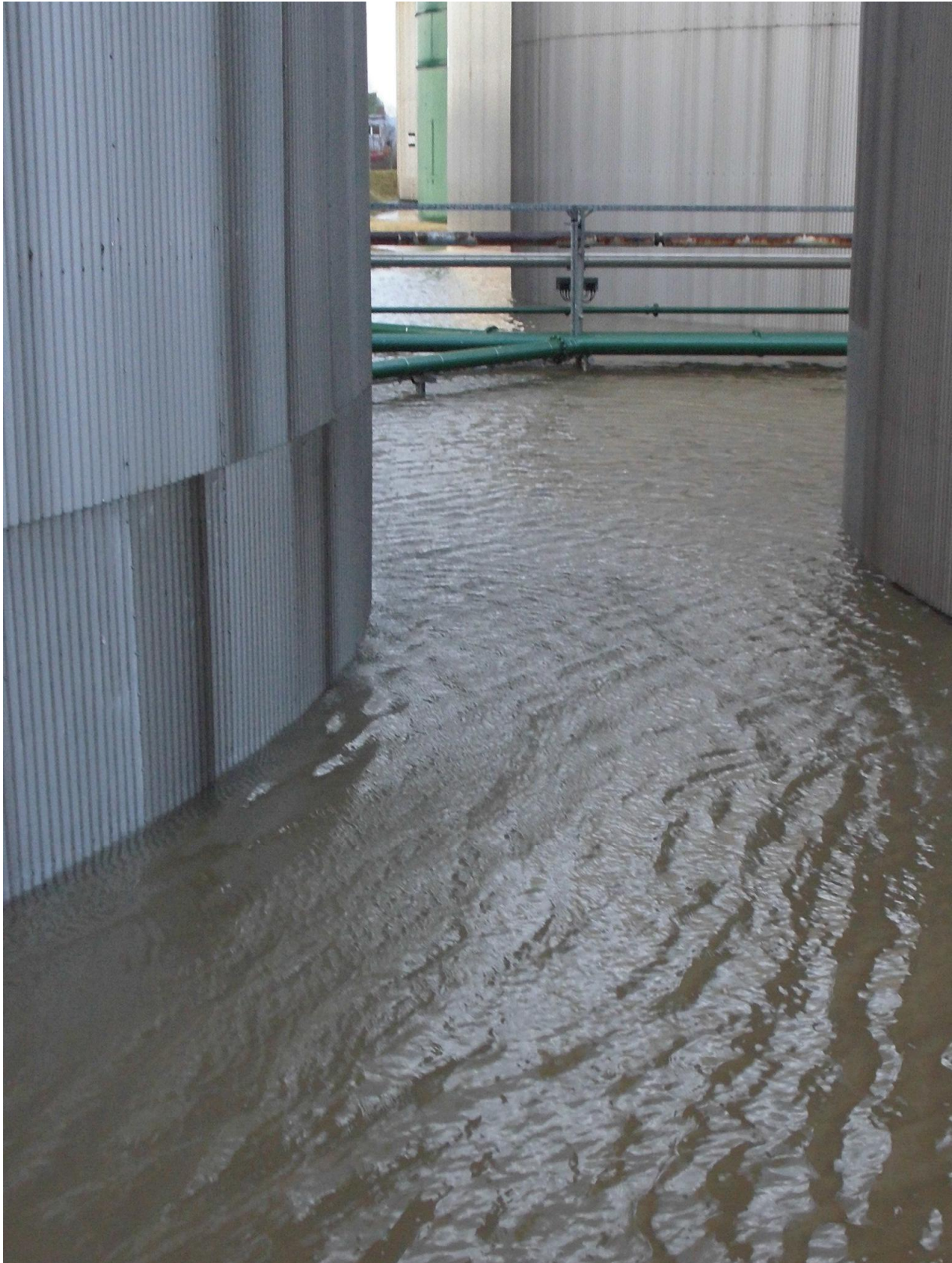
Figure 4 Water inside the tank pit at Terminal Neuhof (water flowed through the tank dike)
