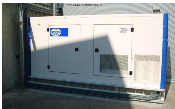
Figure 4-21 Mobile back-up generator
