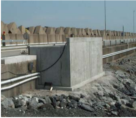
Figure 28: View at the overtopping tank on site.
