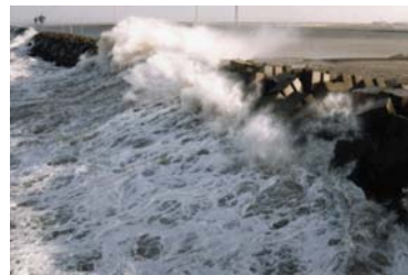
Fig. 3: Wave overtopping over breakwater crest.
