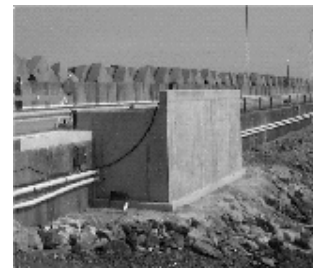
Fig. 4: Overtopping tank behind crest.
