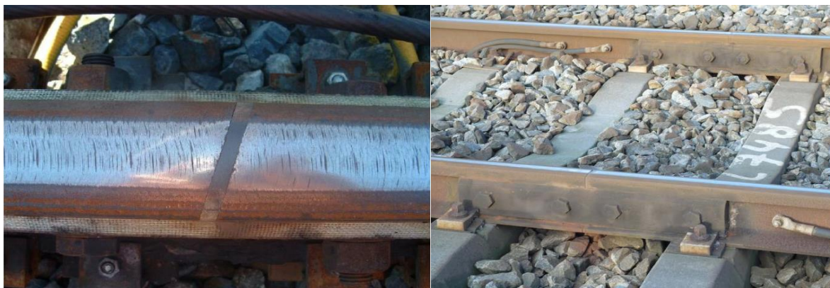
Figure 1.1: (left) IRJ in Australia at 15 degrees (Mandal,2010); (right) square cut IRJ in the Netherlands (ProRail,2019)
