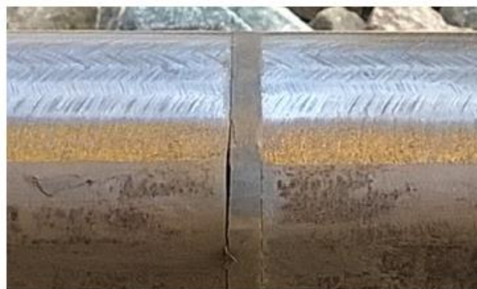
Figure 1.7: Delamination of end post and rail end (J. Bos)
