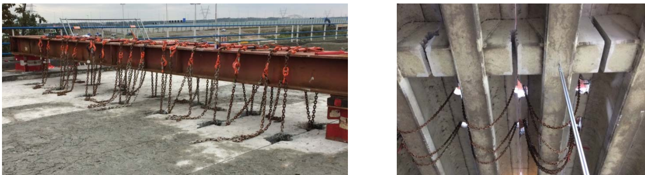
Figure 6 Safety system for single beam tests (steel chains), top side (left), bottom side (right).
