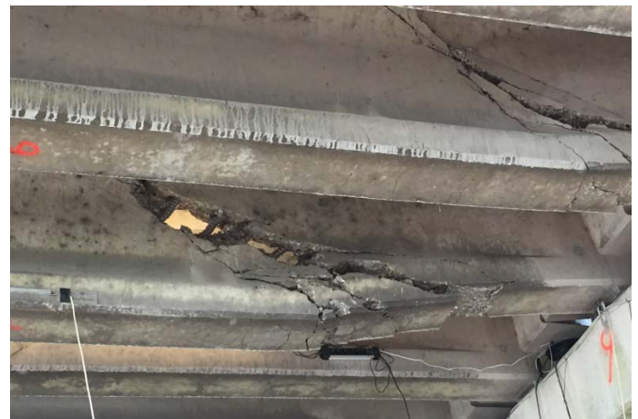
Figure 18 Shear failure beam test 6 and 7
