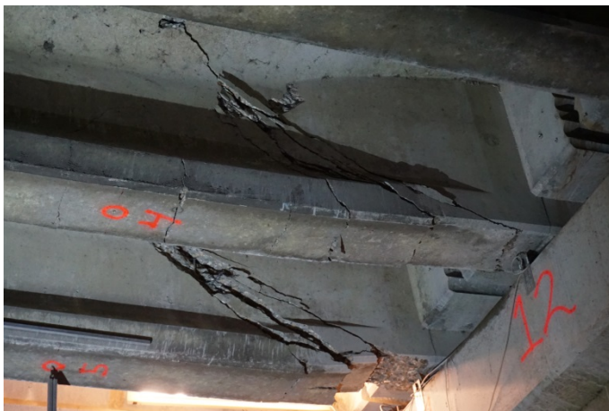
Figure 17 Shear failure beam test 4 and 5
