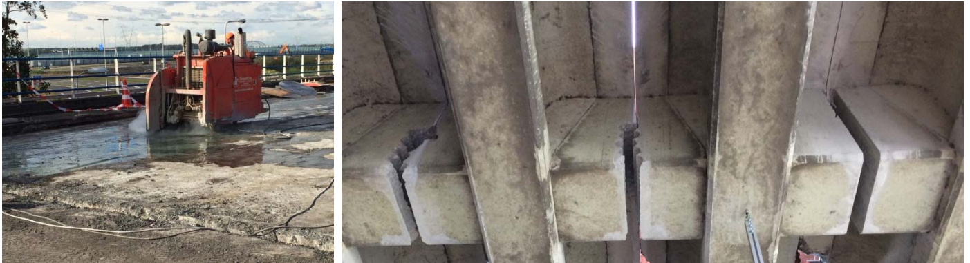
Figure 4 Sawing through the cast-in-between slab (left), sawing and drilling through the cross-beams (right).
