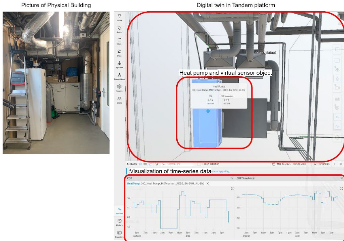
Figure 2. Comparison of the digital twin prototype with the actual building and visualisation of COP.
