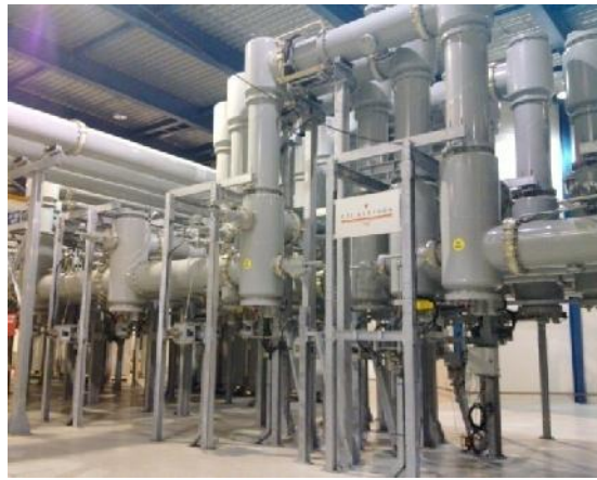
Figure 1.1 Part of the 380 kV gas-insulated substation in Meeden, the Netherlands
