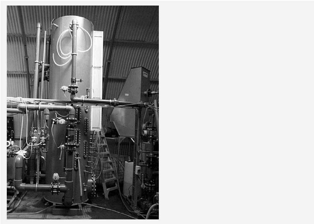
Figure 2.3 Picture of the multi-media filter used in pilot-plant tests
