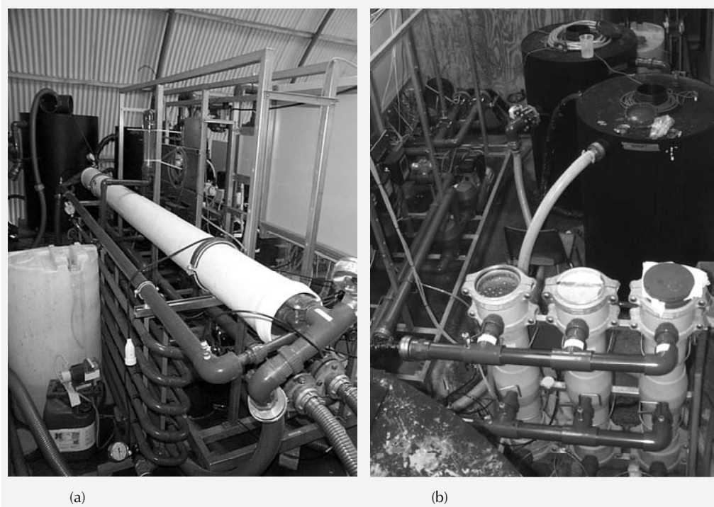
Figure 2.2 Picture of two ultrafiltration membrane modules: (a) horizontally placed module, (b) vertically placed modules in the front
