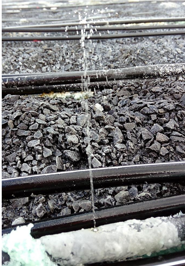
Figure 2. Discharge from an emitter working in a significantly clogged drip line.
