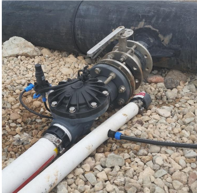
Figure 57. Netafim's flushing and pressure control valve installed on the sub-main pipe. Source: www.aquaroyalspring.com .
