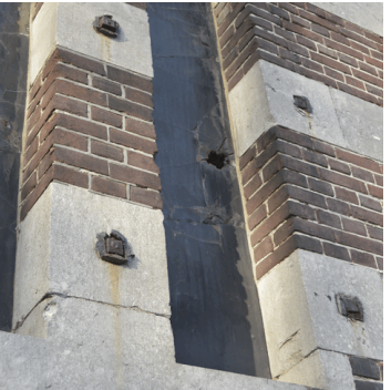
8. traces of removed iron bars.
