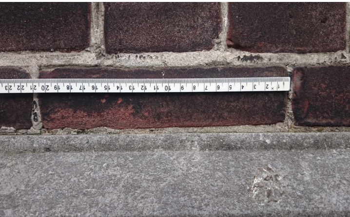
photo 3: width of a full stone is aprox. 210mm
