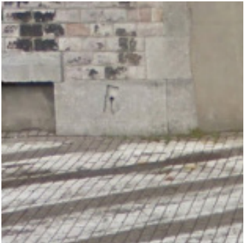
2. traces of an element that was once attached to the wall. possibly the same T-shaped pieces as #1.
