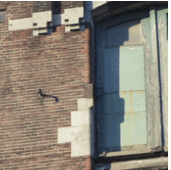
7. Santos had lamps that could be moved to the required loading door, this might be traces of such.
