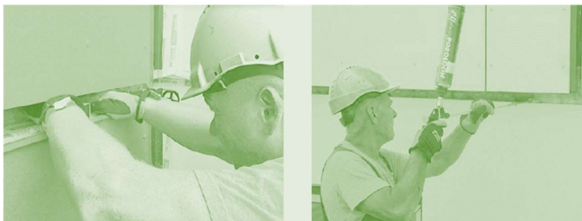
Figure 29, Insulation process with EPS foam after the installation of the façade elements Source: (More-Connect 2019)
