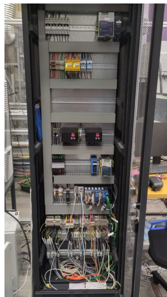
Figure 4.7: Data acquisition and control cabinet holding the cRIO-9067 embedded controller and different NI modules
