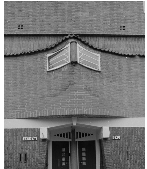
Figure 10. Restoration with wrong bricks. From Collectie Bureau Monumentenzorg: negatiefvellen, by H. van Gool 1990. Stadsarchief Amsterdam
