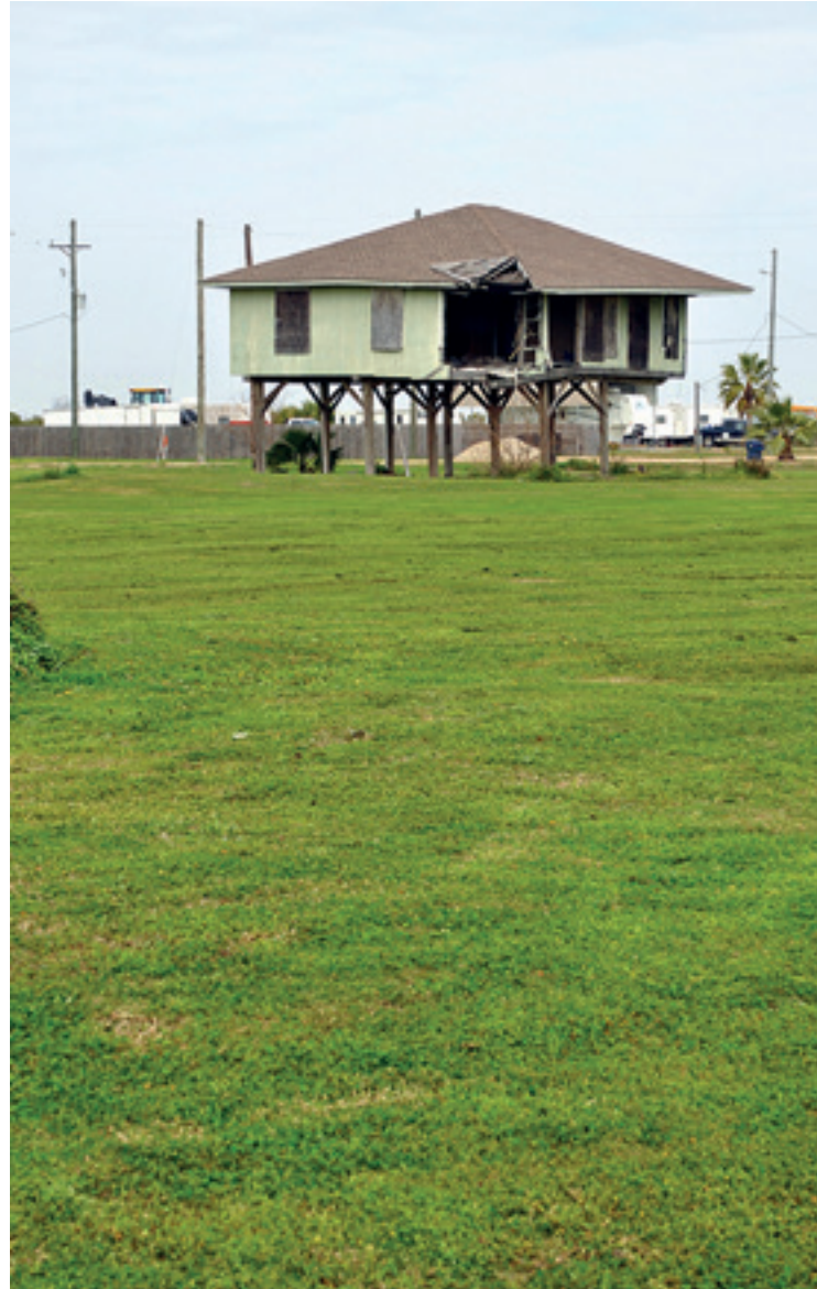
Figure 2. Elevated but still destroyed residence at Galveston Island, never repaired after Hurricane Ike (Photo courtesy Helena Van Boxtelaere).
