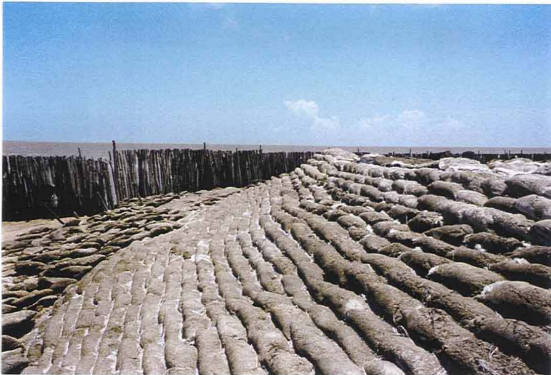
Sandbag revetment in Surinam (Coronie)
