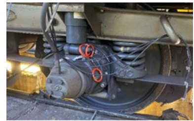
Figure 71-1 The installed ABA system
