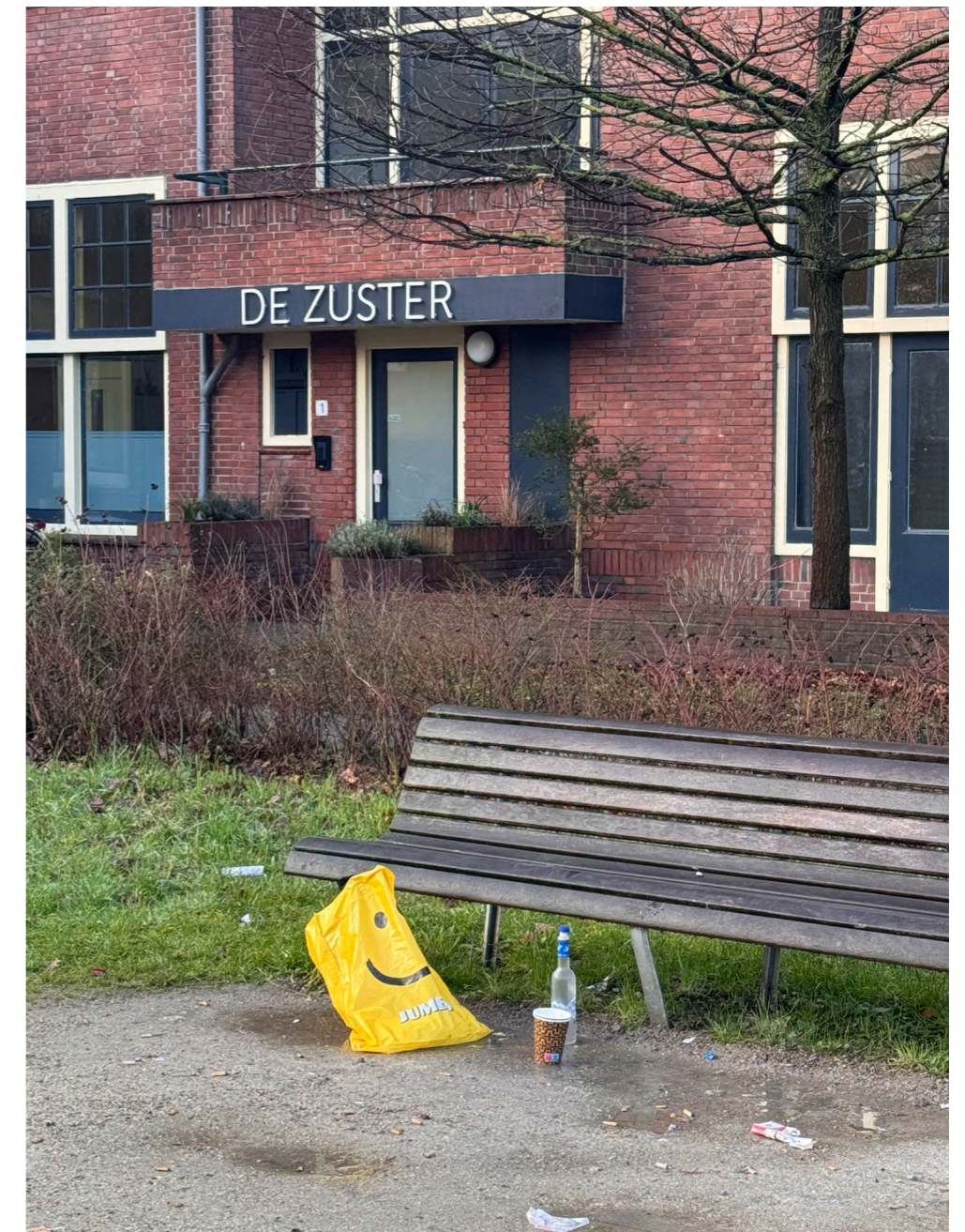
The Zuster, Dilapidation in front of the entrance
