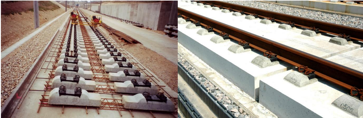
Figure 10 Ties of a Rheda 2000 slab track system before they are casted in the concrete (left) and after casting (right)
