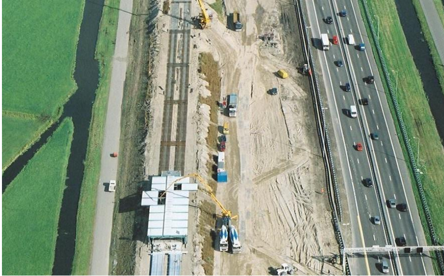
Figure 32 Ditch located parallel to the rail embankment and highway broadening (beeldbank RWS)
