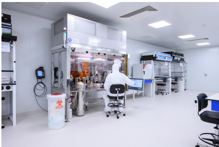
Figure 5.9: Cleanroom/controlled-environment installation. (Dagard, 2026)
