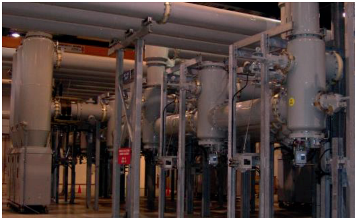
Figure 1-1: Part of a typical 380 kV GIS substation (case study A)
