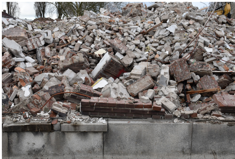
Figure 0.3 | Demolition of housing block at Gardesiaweg, Rotterdam. Piles of material are wasted by demolition practices. (By author, 2026)
