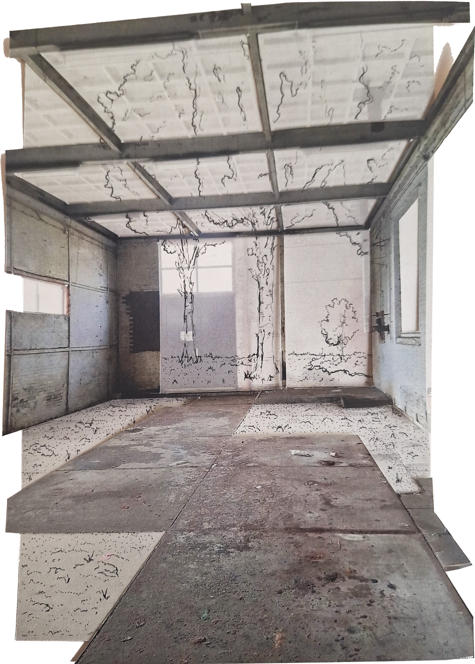
Figure 4.18 | Increased porosity. Removed roof, wall and floor elements open up the space for different uses and processes.
