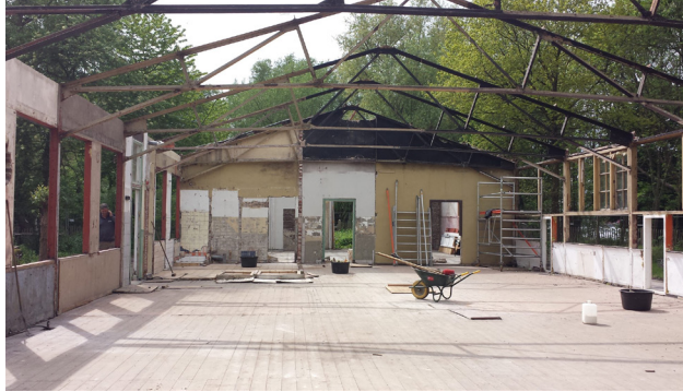
Figure 08 | Construction of Van Brienoord pavilion. Superuse Studios repurposes building materials (Kamphuis, n.d.)
