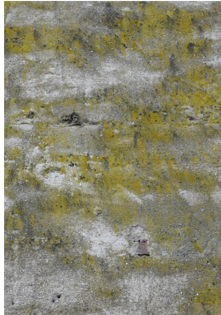
Figure 3.26 | Algae on concrete facade of Keileweg 26-28. Rough material as habitat for growth. (Floor van der Vliet, 2026)
