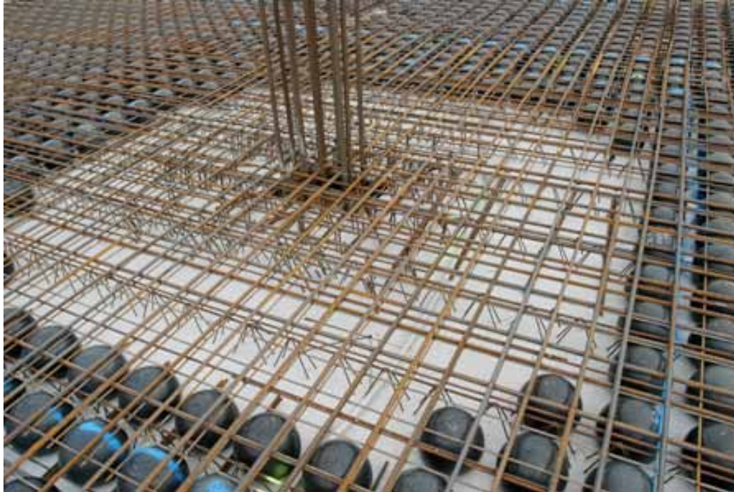
Bubbledeckfloor around a Column. More strenght is needed.
