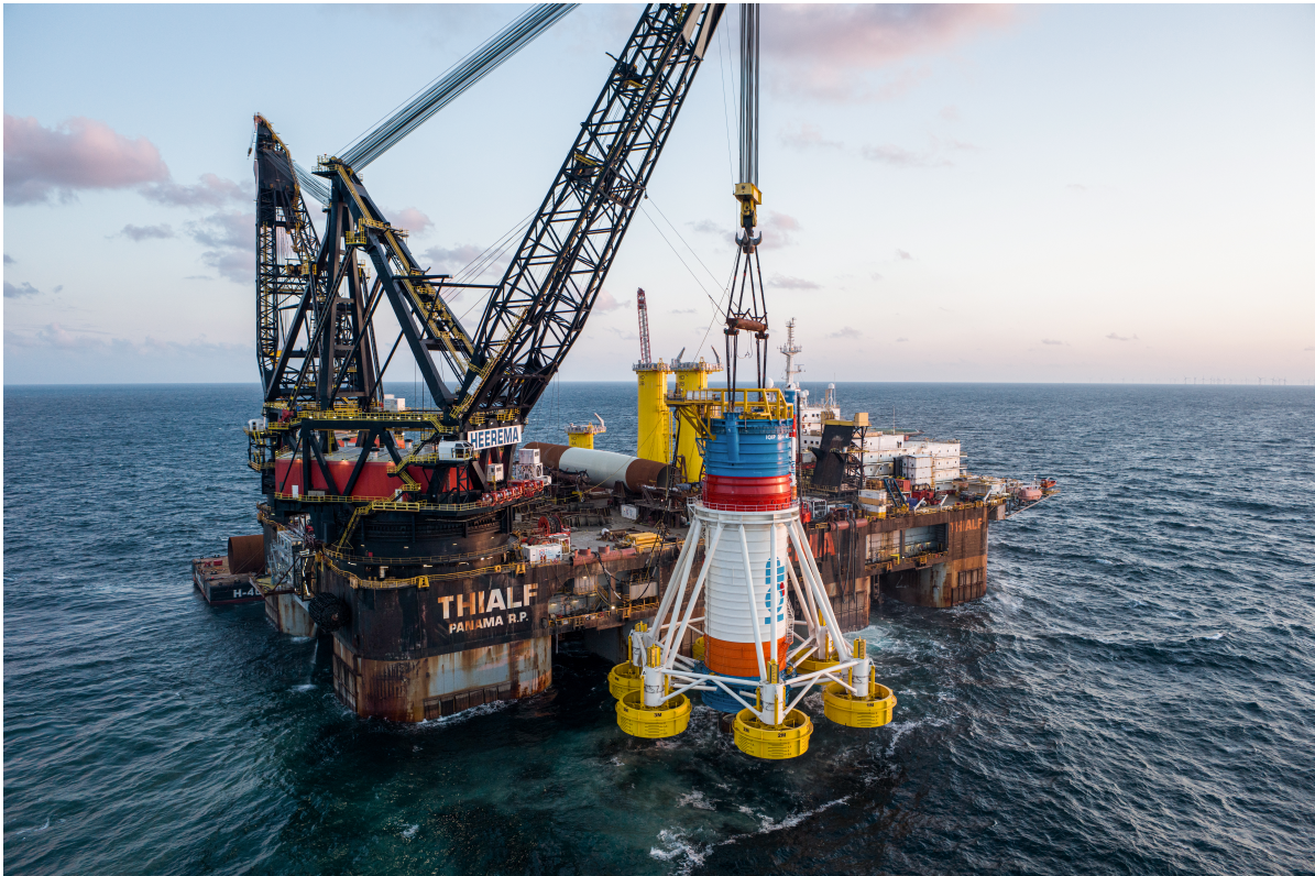
Figure 2.14: Deployment of the NMS from the semi-submersible heavy-lift vessel Thialf during MP installation (Heerema Marine Contractors, 2024b)
