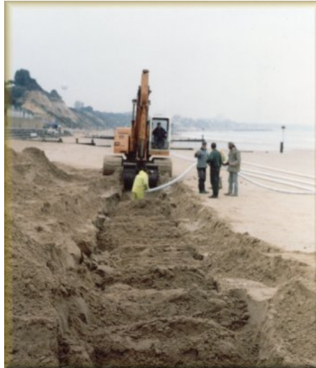
Fig. 2.44. The beach drains may be installed during low water by digging a trench using a backhoe
