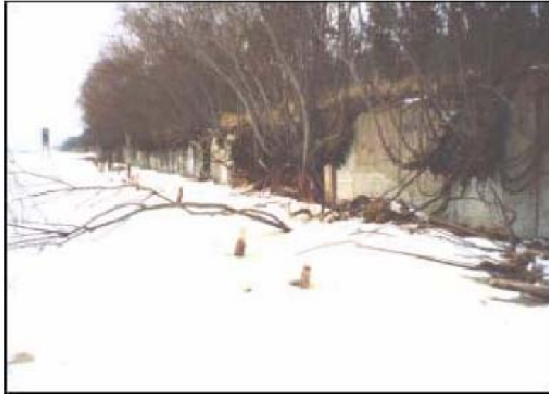
Fig. 359 The concrete base of the foredune, erected after the storm of 1969 and exposed again after the erasure of the foredune in November 2001 (photo: G. Eberhards).
