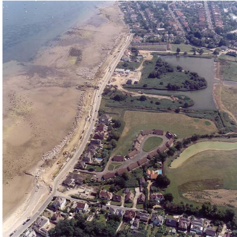
Fig. 3.54. General overview of the Duver site, showing construction work along the beach on the outfalls for Barnsley Brook watercourse.
