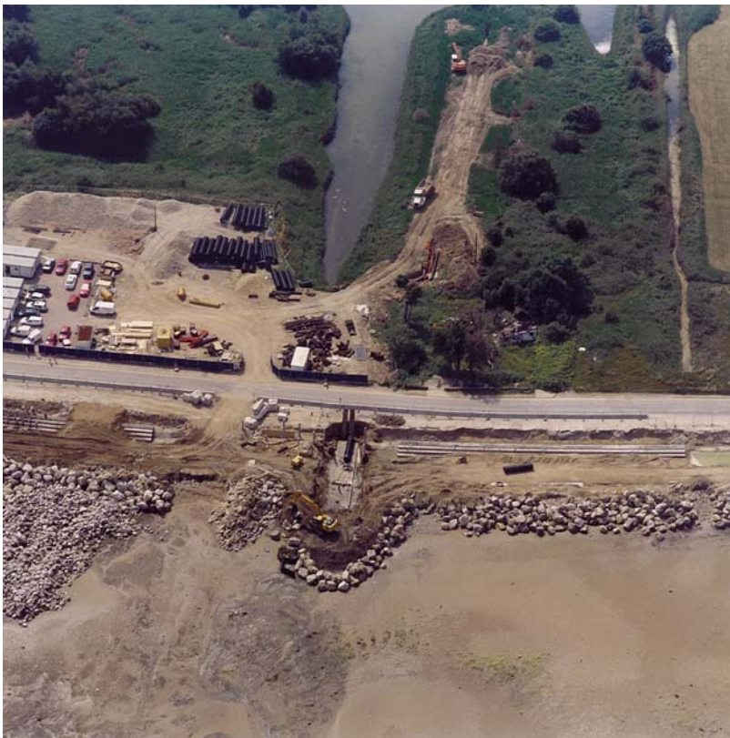
Fig. 3.55. Construction work on an outfall at the western end of the frontage.
