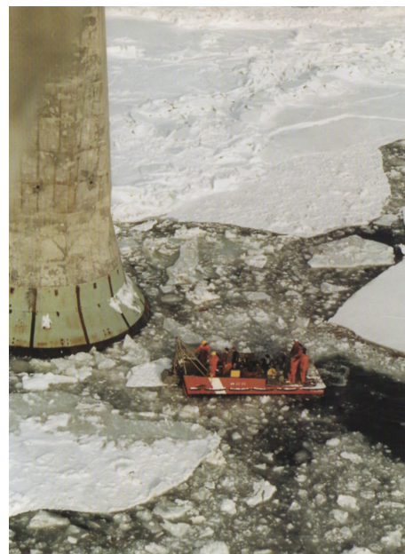
Figure 1.1: Ice pushing against bridge pillar
