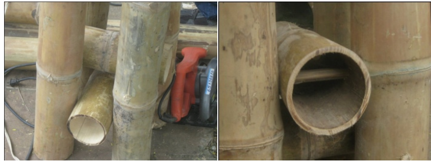
Fig.63 Multi-culm column connection: A standard practice is to add several culms to strengthen the structural capability of one single culm, thus allowing greater loads to be transferred safely throughout the structure.
