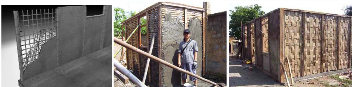
Fig. 45 Grid wall system rendering by Arch Daniel Romero (Paudel, 2007) , Fig. 46 Prototype bamboo housing in Bali, Indonesia (Widyowijatnoko,2010).
