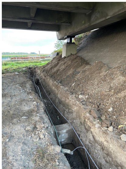
Figure 6.8: The beams discovered during the realization of Lisserweg Viaduct replacement. Retrieved from: www.projecta44.nl
