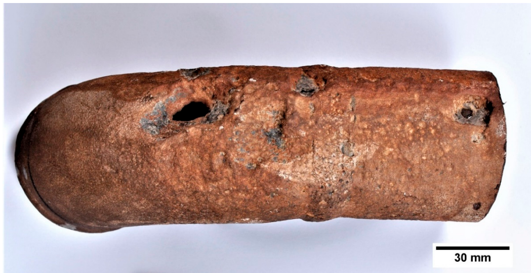
Figure 2. An example of the failed elbows.
