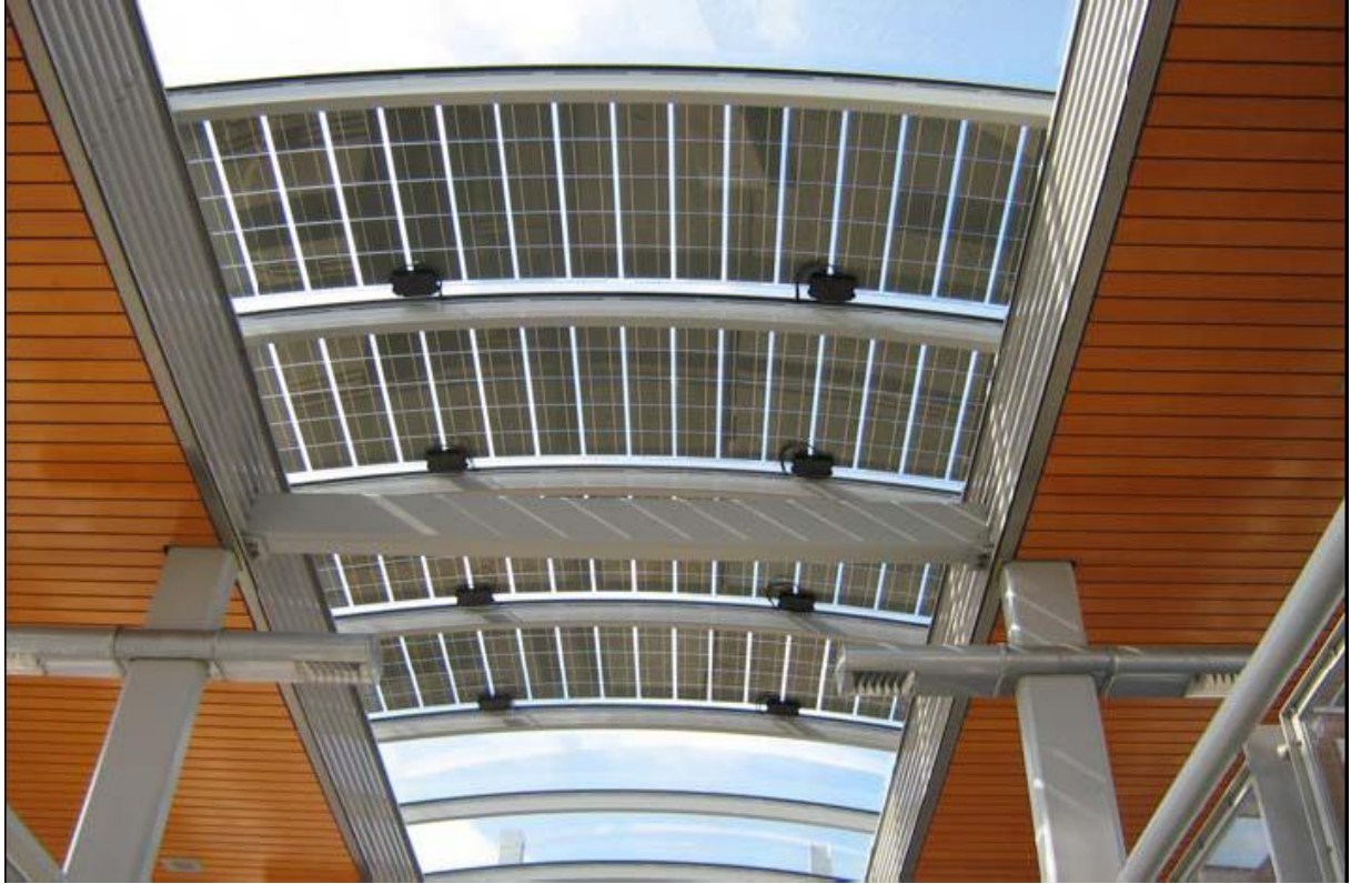
Figure 0-2, Solar panels and freeformglass (Movares B.V. 2008)
