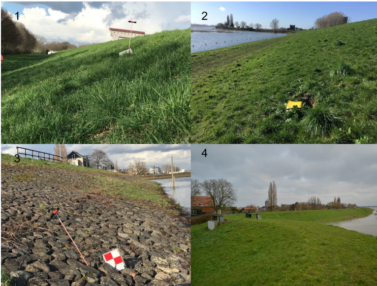
Figure 6.3.: Impression of the 4 sections. Photos for sections 1, 2 and 3 were taken by inspectors during the test. Photo 4 was taken by one of the supervisors. Visible damages are for instance animal burrowing (section 2) and missing joint fill (section 3).
