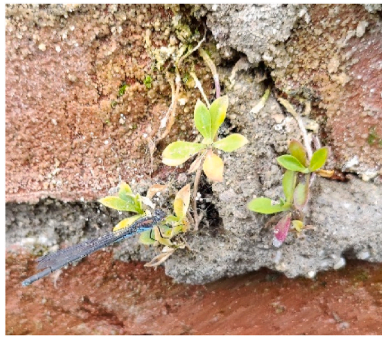
Fig. 11. Wallflower growing in the cracks present in a rough mortar joint.
