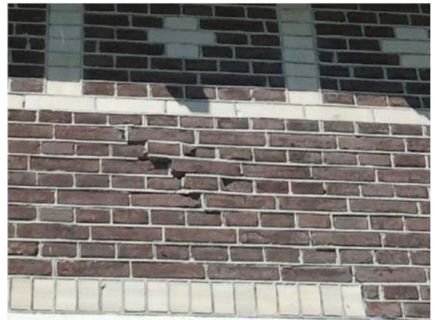
Figure 109: Loose masonry at the location of floor beams caused by beams, www.namplatform.nl
