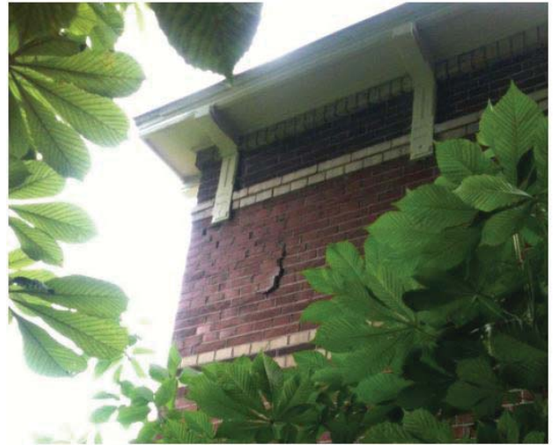
Figure 108: Loose masonry at the location of floor beams caused by beams, www.namplatform.nl
