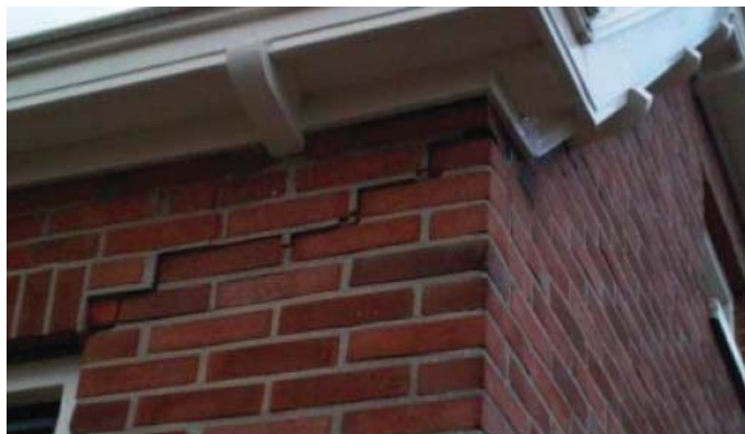
Figure 5: Earthquake damage, source: www.groninger-bodem-beweging.nl
