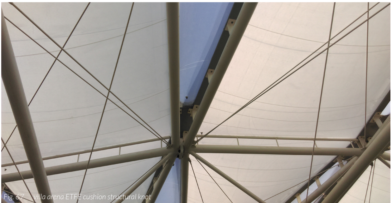
Fig. 66 villa arena ETFE cushion air supply
