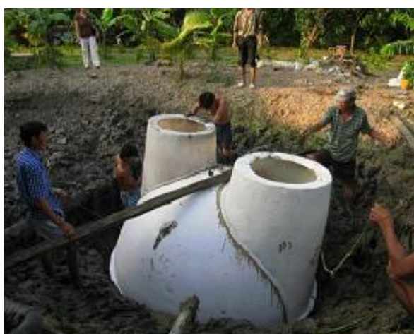
Figure 4.16: Installing prefabricated biogas digester at a project site in Vietnam. Retrieved from: [24]
