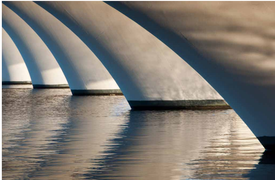
FIGURE 2.11 Daylight underneath the bridge increases due to the void between the decks. Royal HaskoningDHV, Joris Smits et al. (2013). Photo by Elroy Blom 2012.
