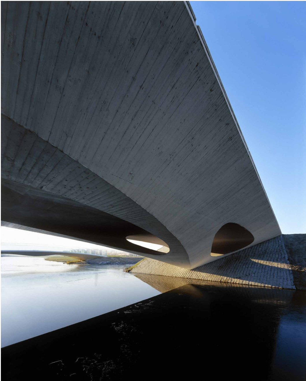
FIGURE 3.8 View on the intersecting cavities in the abutment on the water side. Clearly visible are the rough timber planks in the formwork of the vault and the sides. The cavities are smooth inside. Royal HaskoningDHV, Joris Smits et al. (1999). Photo by Bart Nijs 2004.
