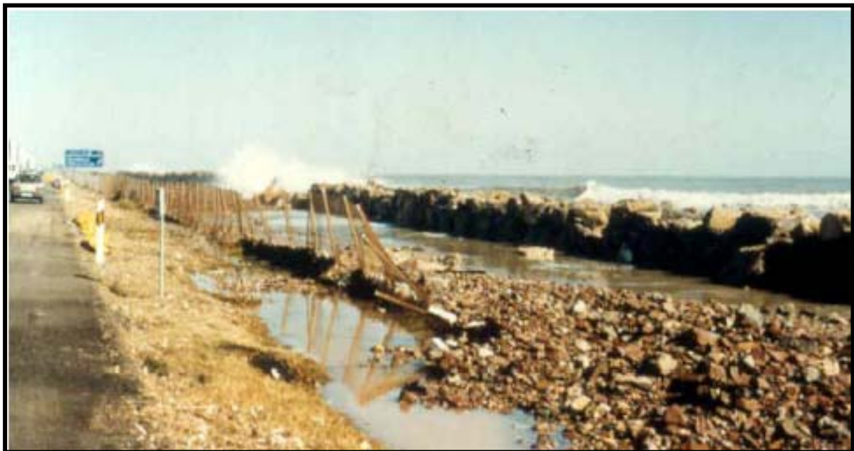
Figure A2.3. Damages on the motorway coastal defence.
