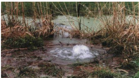
Figure 1-2 the outflow of seepage water, but no piping (TAW, 1999)
