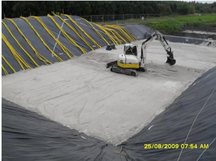
Figure E-3 the construction of the sand layer in de IJkdijk (de Bruijn, 2009)
