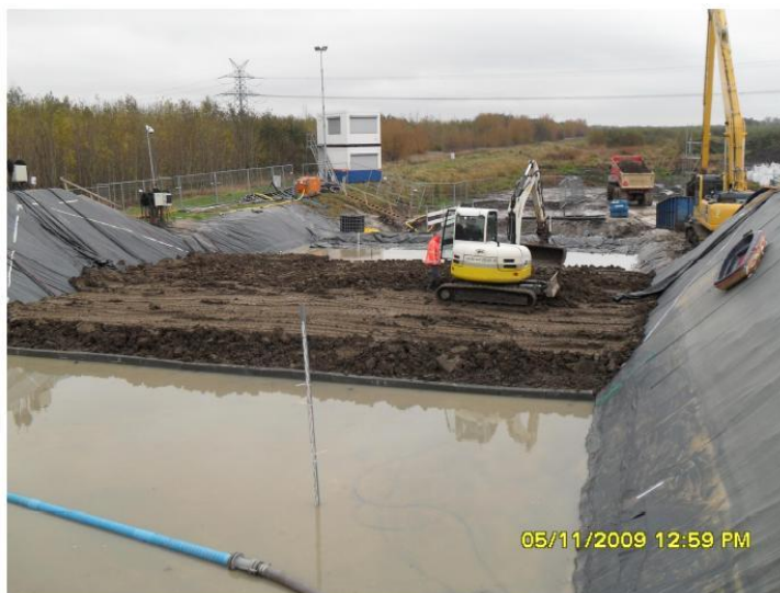
Figure E-4 the construction of the clay dike in de IJkdijk (de Bruijn, 2009)
