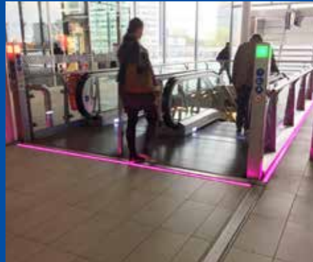
LED-line along all access points from the hall to the platform (Utrecht CS).
