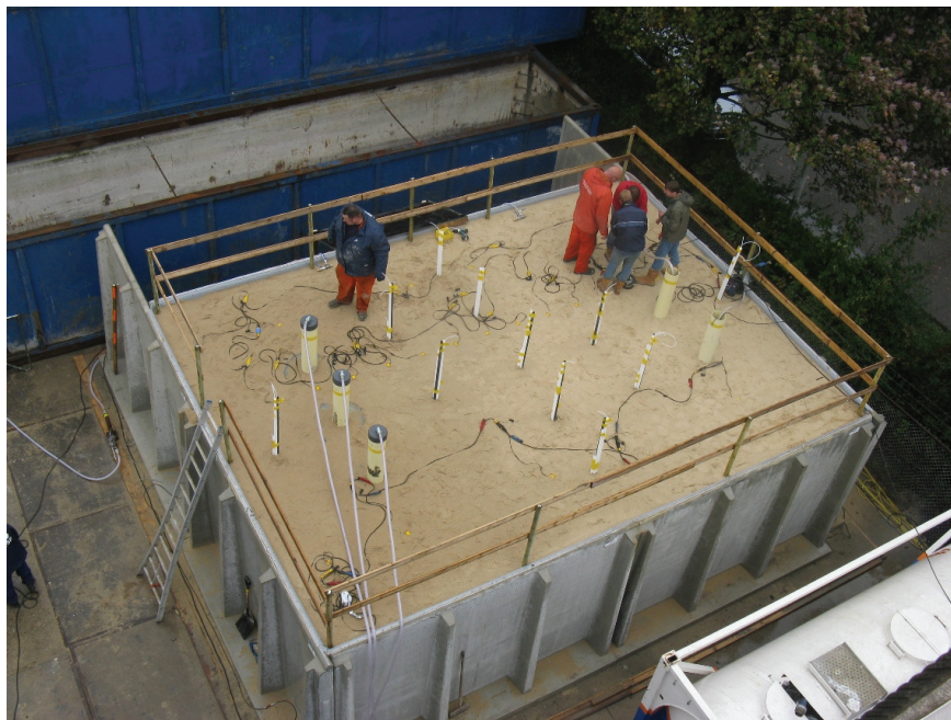
Figure 5 set-up for large scale Biogrout experiment ( 100\text{m}^3 ). Three injection wells (left) and three extraction wells (right) were used to flush liquids through the sand body.
