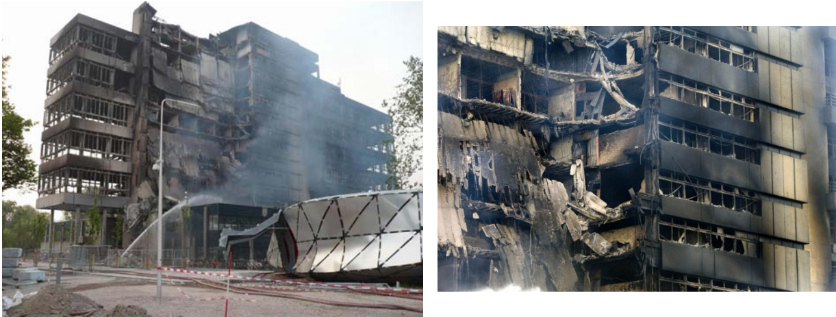
Fig. 1.6 Damage to the concrete multi-storey building of the Faculty of Architecture at Delft University of Technology in the Netherlands after the fire on May, 13 th 2008 (pictures by ANP).
