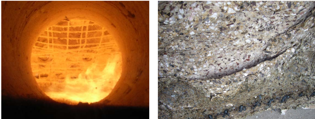
Fig. 1.11 The high temperatures reached during the fire test can cause the exposed reinforcement to melt (left) (picture by MFPA 3 ). After the fire test a partially detached surface layer was observed at the centre of the tunnel lining segment (picture taken at the MFPA 4 ).
