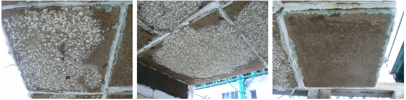
Fig. 2.27 Spalling damage of B60 or C60/75 slabs after exposure to a fire corresponding to the HCinc curve. The slabs were stored at ambient conditions without (left) and with addition of 1.84 \text{ kg/m}^3 PP-fibres (middle) or predried at 80^\circ\text{C} (right) (Pictures by Mindeguia 8 ).
