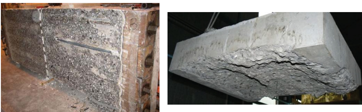
Fig. 2.25 Spalling as observed during exposure of compression loaded C35/45 slabs to a RWS type of fire (left) (Jansson & Boström, 2008). Exposure of a B60 or C60/75 slab to a low heating rate still causing spalling (right) (Mindeguia, 2009).
