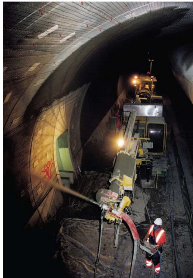
Fig. 1.15 Spraying of heat resistant cladding in the Western Scheldt tunnel in the Netherlands (Heijboer, et al., 2004).
