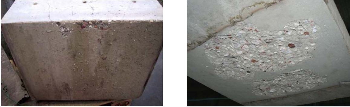
Fig. 2.24 Exposure of a water stored C25/30 (left) (Horvath, et al., 2004) and an air stored B40 or C40/50 (right) (Mindeguia, 2009) slab to an ISO type of fire indicating only for the latter one limited surface spalling, attributed to the flint aggregates.
