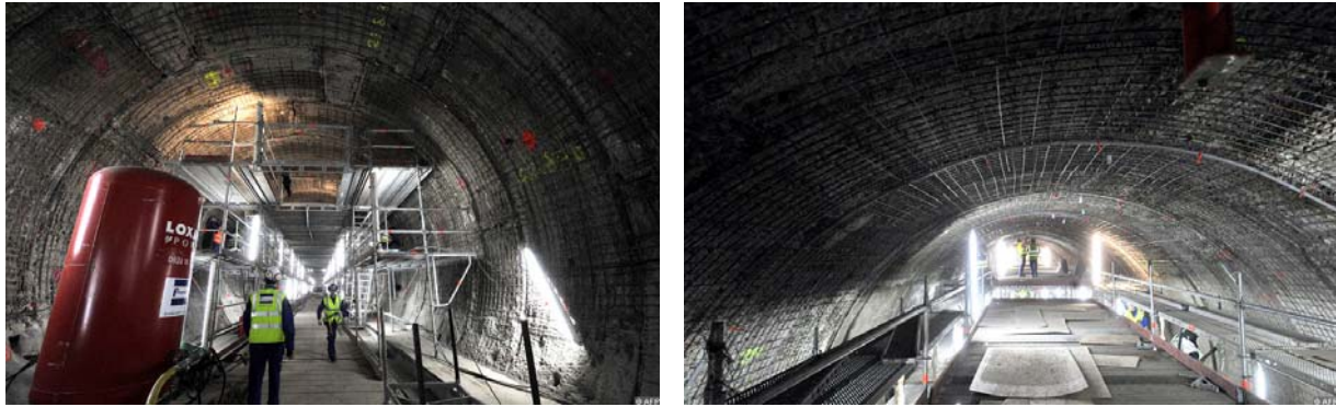
Fig. 1.7 Damage and repair works to the Channel tunnel between France and England after the fire on September, 11 th 2008 (pictures by AFP).
