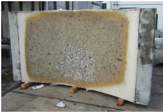
Fig. 1.14 Tunnel lining segment with PP-fibres after full-scale fire testing (picture taken at the MFPA 5 ).
