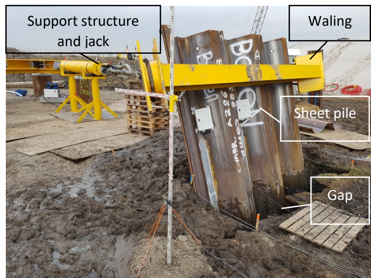
Figure 4.26 PO-test on triple AZ26 panel, with pushed up soil on front (passive) side and gapping on back (active) side.
