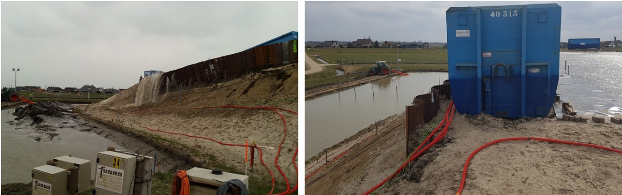
Figure 4.36 Left: Side view of failure deformations at the moment of flooding. Right: Top/side view of the SPD prior to failure.
