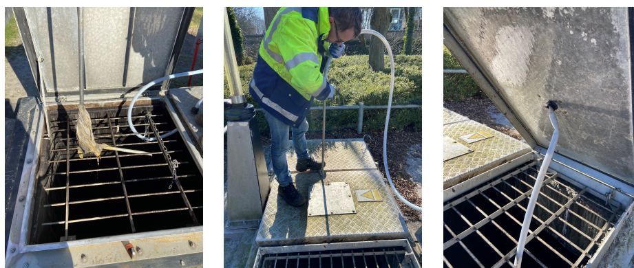
Figure 9.5: Images of mechanical errors during a visit to samplers at three pumping stations. In the left picture the contamination of the suction pipe by wipes is visible. In the middle picture, the angle of the suction hose is adjusted so it could be placed back in the proper position relative to the direction of flow in the pumping station. In the right picture it is shown that the suction pipe, connected to the sampler, was clamped.
