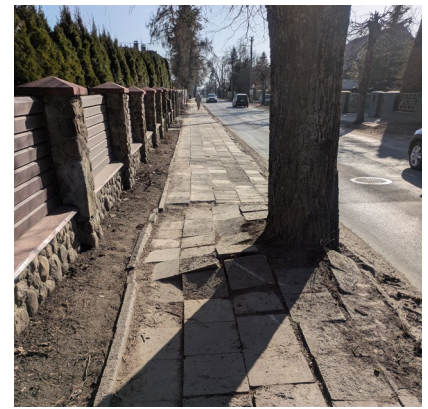
85. Pedestrian tripping hazard.
