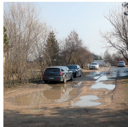
92. Potholes and puddles in Riešè, VDM.
