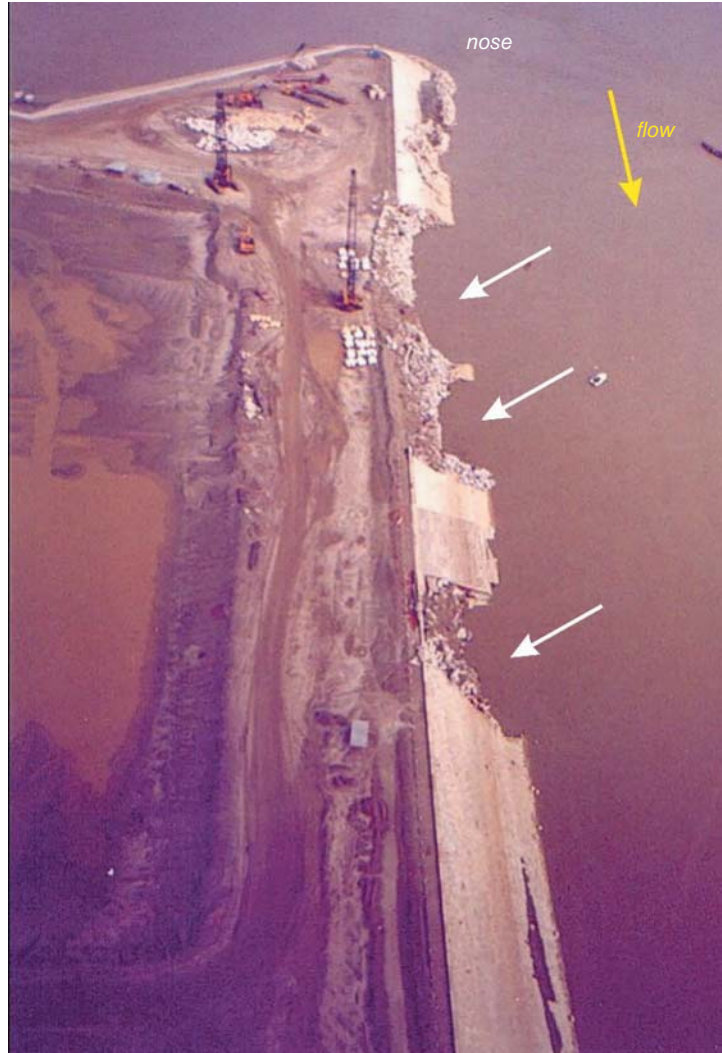
Figure 20.34 Image of the B2 hardpoint in 1998 showing the multiple failures (white arrows) formed at the height of the 1998 flood. Flow towards viewer and the upstream nose of the B2 hardpoint is labelled. Source: Photograph courtesy of Mr. Bob Courtier, W.S. Atkins Ltd.
