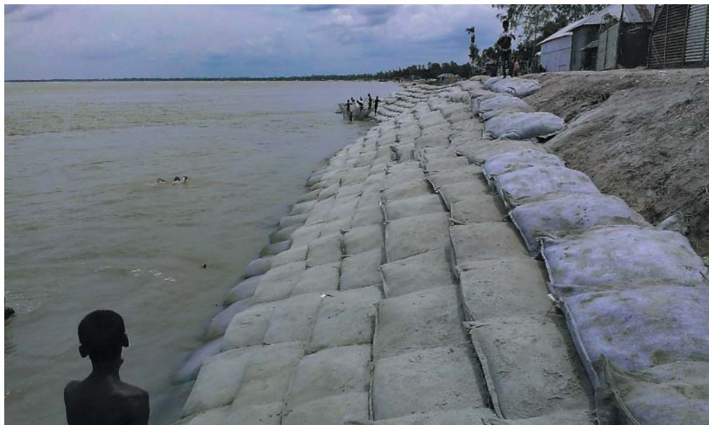
Figure 20.35 Sand-filled geotextile bags, or geobags, used for bank protection at Chauhali, Jamuna River. View looking upstream.
