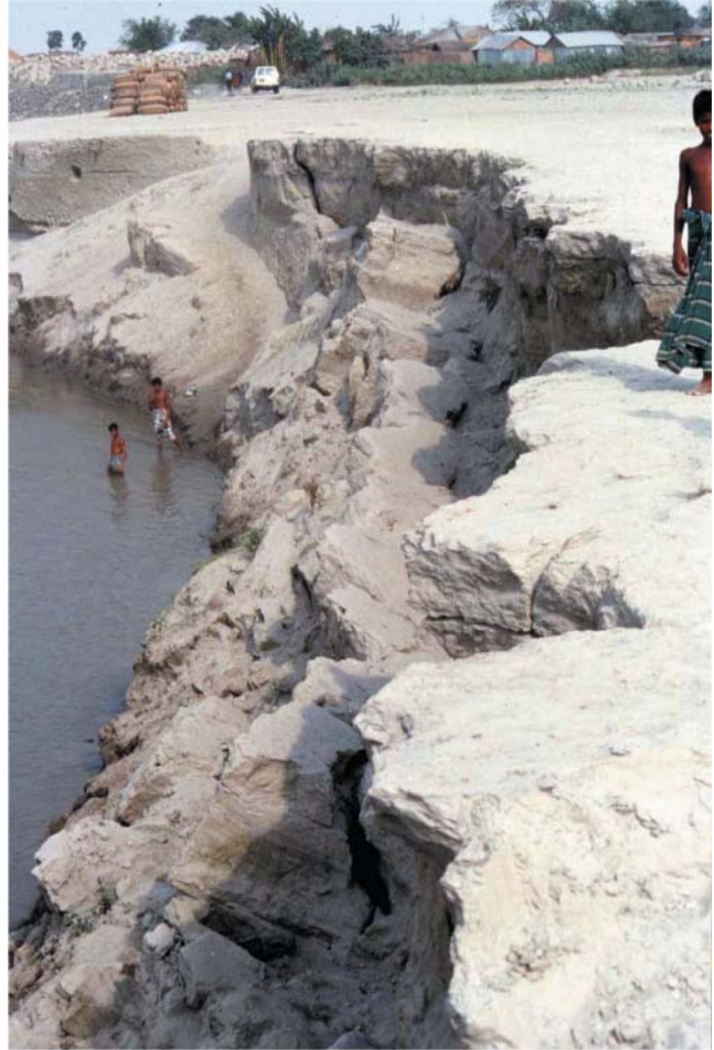
Figure 20.29 Large-scale slab failure by bank undercutting near Shailabari (~4 km upstream of Sirajganj). Photograph taken at low flow. During seasonal floods, the water level would be up to bankfull.
