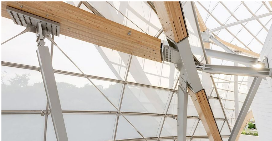
Figure 2.5: Complex hybrid steel-timber joints in Fondation Louis Vuitton. Adapted from HESS TIMBER (n.d.). https://www.hess-timber.com/en/references/detail/museum-fondation-louis-vuitton/
