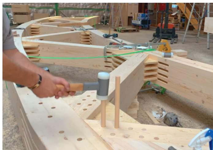
(b) Full timber connection detail of the Luftschiffhalle Mülheim. Screenshot adapted from YouTube (n.d.). https://www.youtube.com/watch?v=Q9WgnQp_JY
