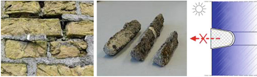
Fig. 4 Detachment of repointing caused, in particular, by thermal deformation enhanced by a wrong cross-sectional form (V-shape instead of rectangular) of the repointing
