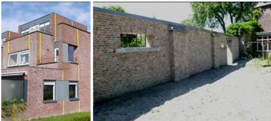
Fig. 3 Left, the yellow lines indicate the dilations applied in a modern masonry. Right, a wall without dilation in traditional masonry (Color figure online)
