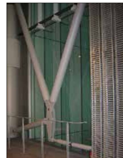
Figure 3.9 MR damper in structural component, Nihon-Kagaku-Miraikan museum, Japan. Image courtesy unknown.
