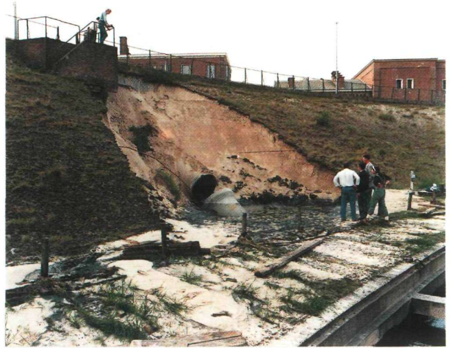
Figure 2 Drinking water pipeline fracture. Detail showing joint with insufficient tensile strength.
