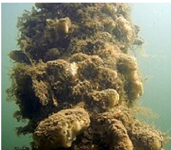
(a) Severe biofouling on a submerged pipe.
